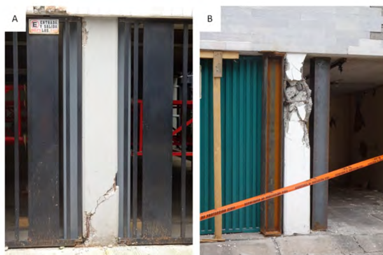
Figure 3.9: (a) Failure of the column in shear. (b) Buckling of the longitudinal reinforcement bars.
