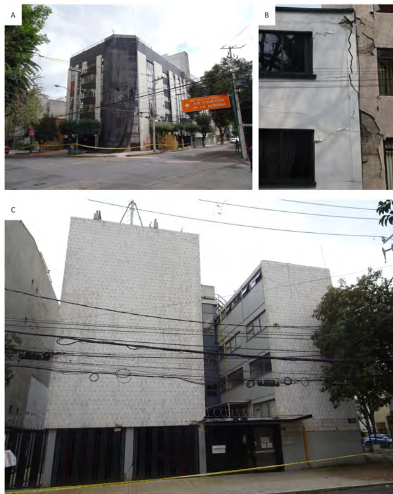
Figure 3.8: Representative damage in La Morena. (a) Corner building with torsion eccentricity. (b) Pounding failure. (c) Soft storey in the ground floor.
